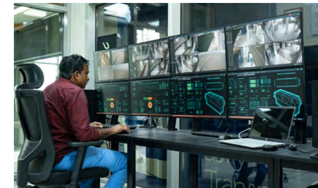
Automated Control System (a set of hardware and software to ensure the functioning of the complex)
